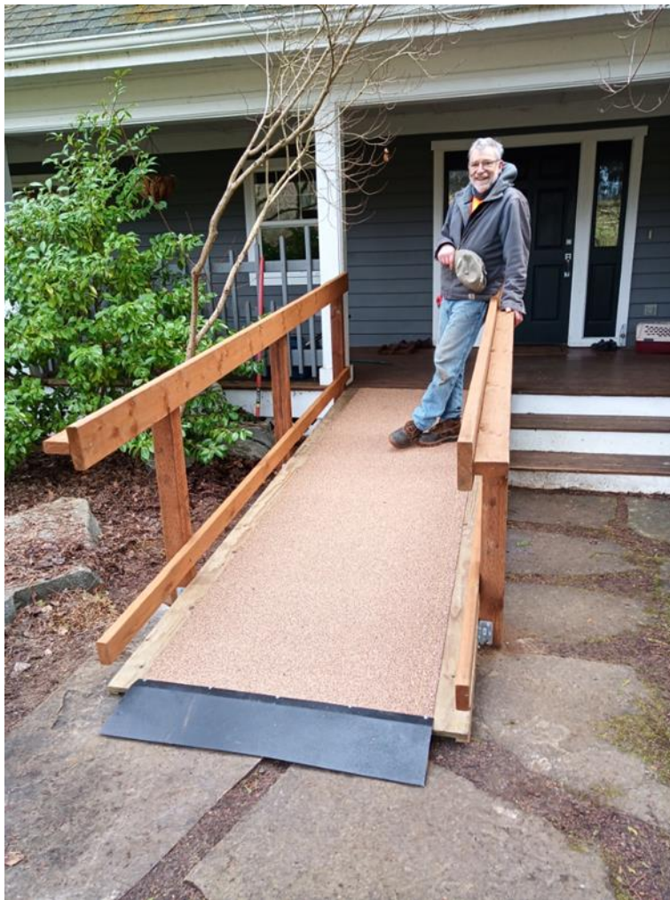
Michael Crovitz with the completed ramp (John White was taking the photo)
